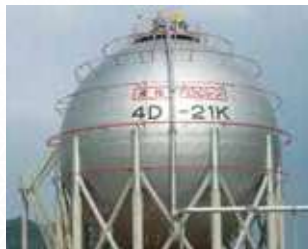
Pressure Tanks (Spherical Tanks)
